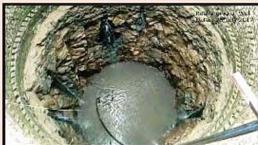
Recharge Well - Mahakal
